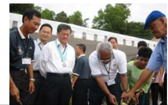
DGE Ivor pouring the cement into the fiberglass mould while DG David Tong & President Sylvester observed with keen interest.
